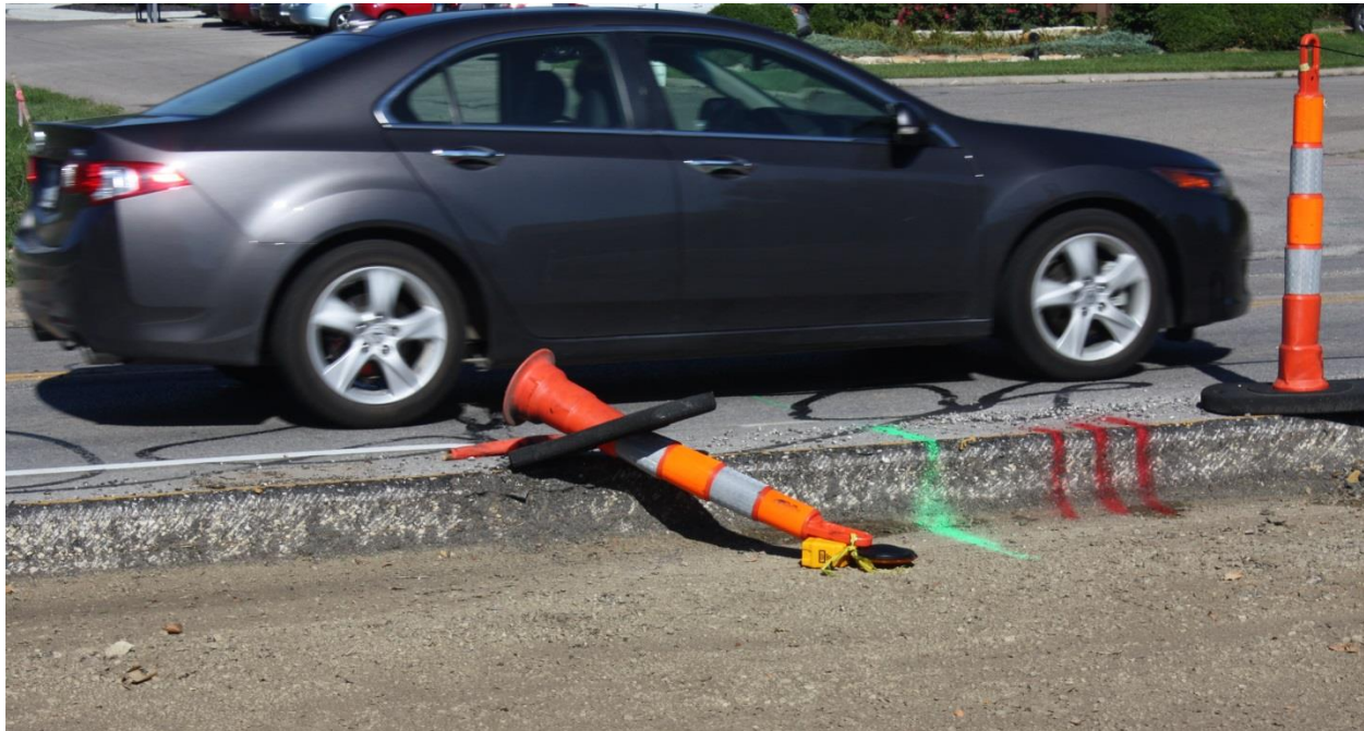
Figure 42. Location 3 Intellicone Sensor on Ground
